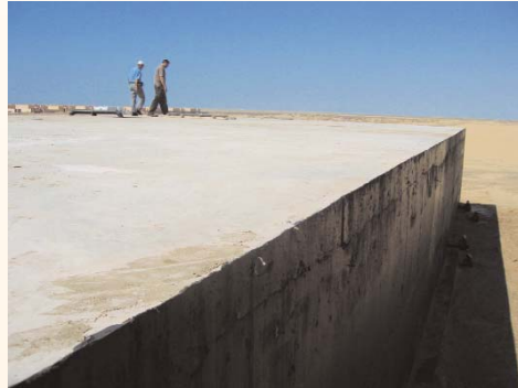
Water storage reservoir at the NPC demonstration site.
