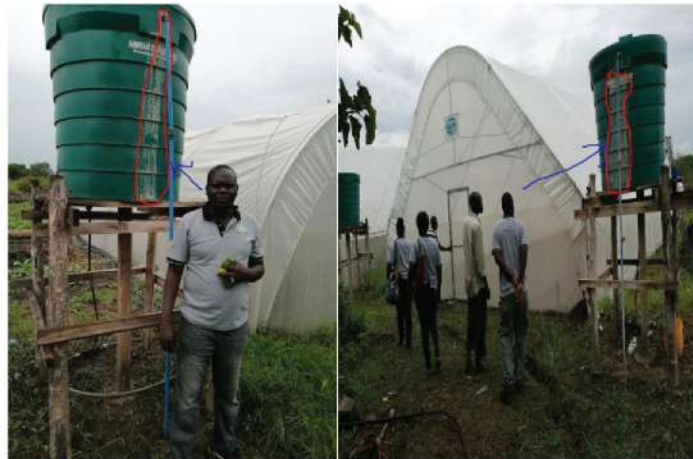
Drip irrigation system for saline groundwater at Juba
